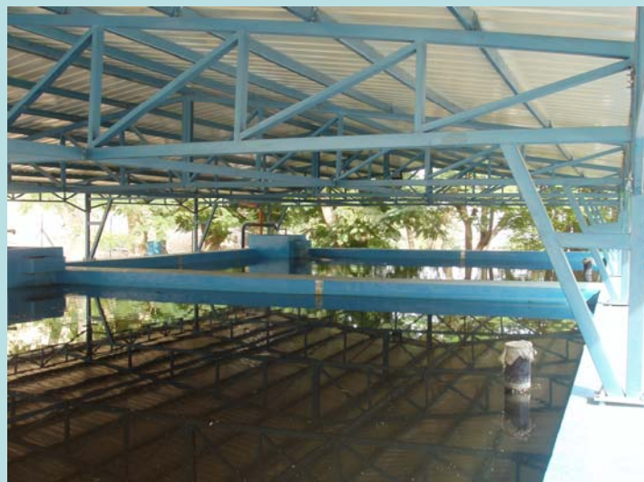
Slow Sand Filtration (Water treatment plant Aqbat Jabr)
