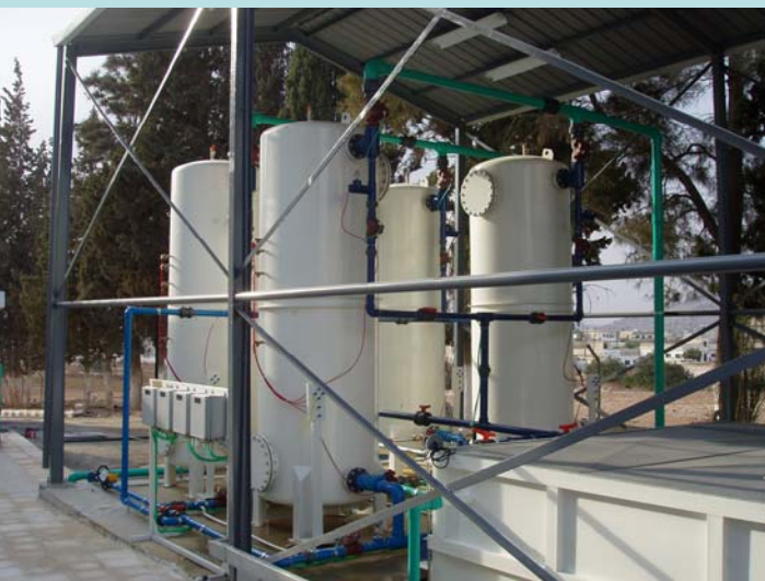
Rapid Sand Filtration (Water treatment plant Baq'a)
